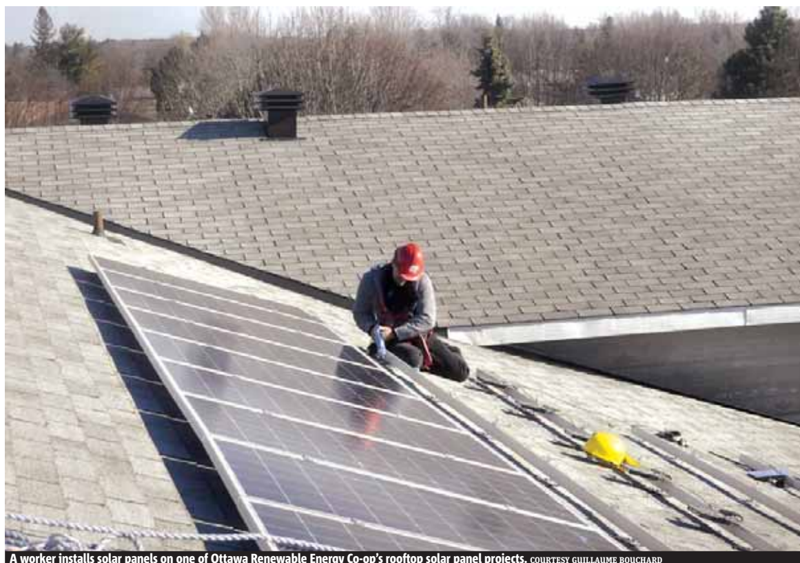
A worker installs solar panels on one of Ottawa Renewable Energy Co-op's rooftop solar panel projects. COURTESY GUILLAUME BOUCHARD
